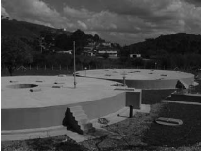
Figure 5.3. Anaerobic filter after upflow anaerobic sludge blanket (UASB) reactor (source: Colombo WWTP, SANEPAR/ Brazil)
