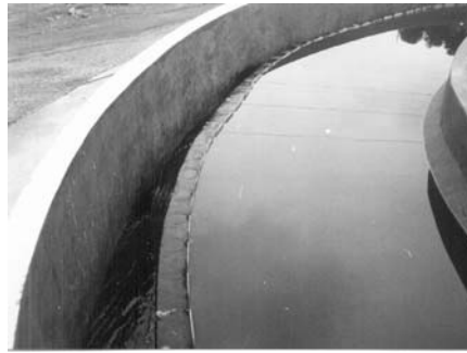
Figure 5.19. Effluent collection device (plate with V-notch weirs) Source: Nova Vista WWTP, Itabira, Minas Gerais, Brazil
