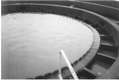
Figure 5.16. Influent distribution structure in a circular reactor (source: Nova Vista WWTP, SAAE Itabira, Minas Gerais, Brazil)
