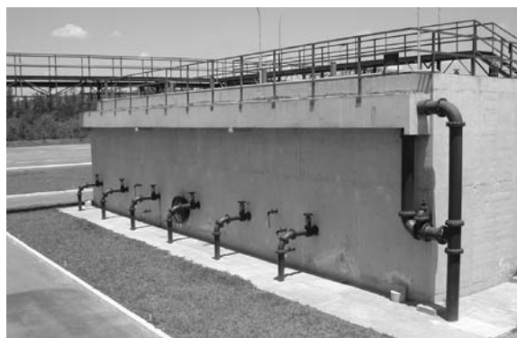
Figure 5.10. View of a full-scale UASB reactor Source: Ipatinga WWTP, COPASA, Brazil
