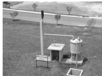
Figure 5.21. View of a hydraulic seal and gas burner (source: Ipatinga WWTP, Minas Gerais, Brazil)
